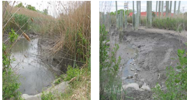
A silted drainage ditch is believed to exacerbate flooding issues upstream near the Post Office and Port Mahon Road.
