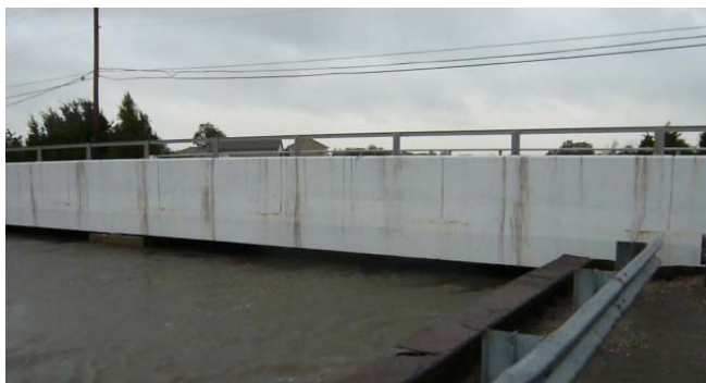
Water level during a 2010 nor'easter nearly reaching the Little River Bridge deck.
